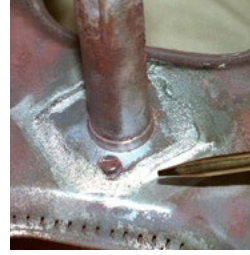
Pyro-Putty® 653 seals corroded burner manifold.
